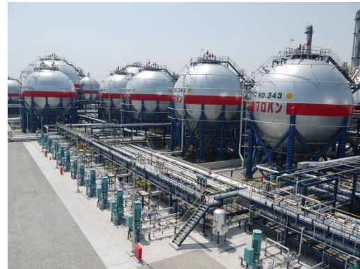
LPG tanks newly installed at Chiba Refinery
