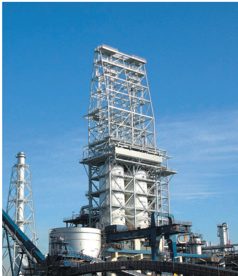
Delayed Coker (Sakai Refinery)
