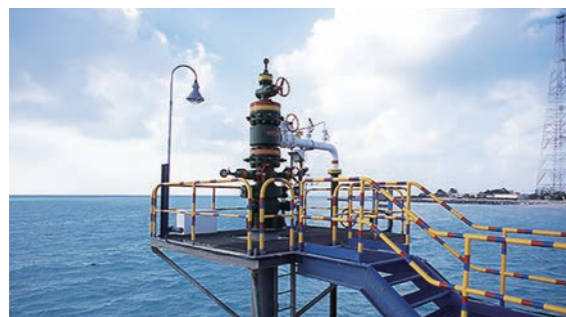
Water disposal well for wastewater injection to subsurface
