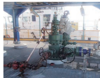
Wastewater injection well and cuttings injection well (zero-discharge operation)
