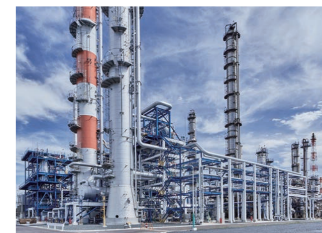
Propylene rectifying tower
