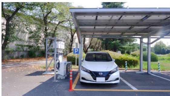
Solar carport, storage battery, EV, and charging equipment installed at the Research & Development Center
