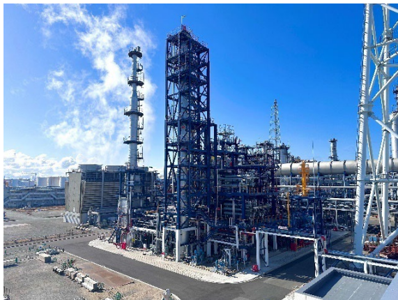
Completed SAF production plant
