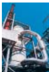
Dioxin removal unit
