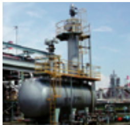
Vapor recovery unit that prevents the release of hydrocarbon vapors into the atmosphere
