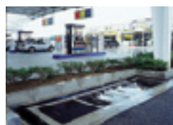
Oil-water separation unit, where oil is removed from water and water pollution prevented
