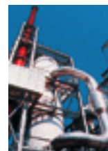
Dioxin removal unit
