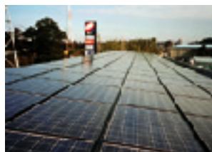
Service station equipped with solar panels
