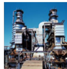
Fuel gas denitration unit which removes NO x from exhaust gases
