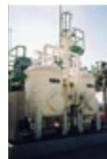
Hydrocarbon vapor recovery unit
