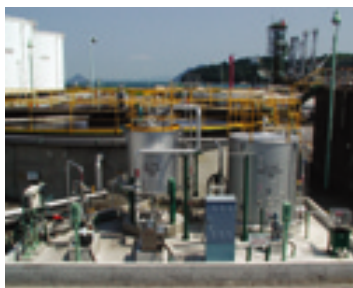
Wastewater treatment unit
