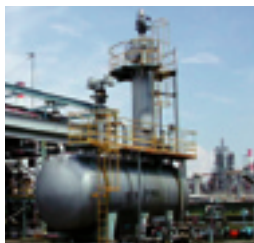
Vapor recovery unit that prevents the release of hydrocarbon vapors into the atmosphere
