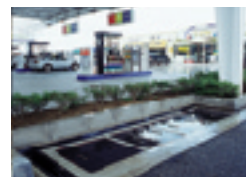
Oil-water separation unit, where oil is removed from water and water pollution prevented
