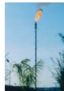
Flare at Balikpapan refinery, Indonesia
