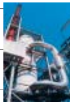
Dioxin removal unit for exhaust gases
