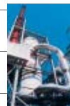
Dioxin removal unit for exhaust gases
