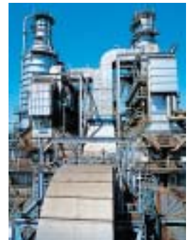
Flue gas denitrification unit removes NOx emissions
