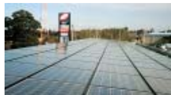
Solar panels at a service station
