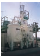
Hydrocarbon vapor recovery unit
