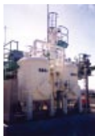
Hydrocarbon vapor recovery unit
