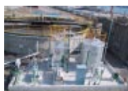
Excess sludge reduction unit
