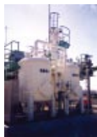
Hydrocarbon vapor recovery unit
