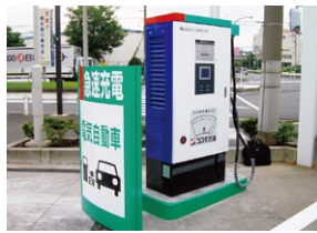
High-speed EV battery recharger
