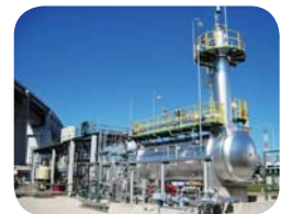
VOC recovery equipment
