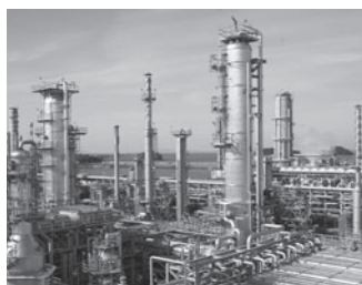
Para-xylene (PX) manufacturing facilities
